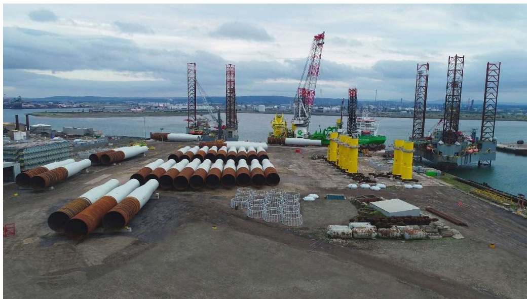
Turbine pre-assembly will take place at Able Seaton Port near Hartlepool, creating 120 jobs during construction.
